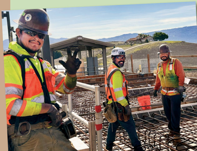
Workers install rebar for new filtration basins at the West Hills Water Treatment Plant (see story on page 1). The expansion will allow us to treat more water during wet years so we can store it for use during times of drought.
